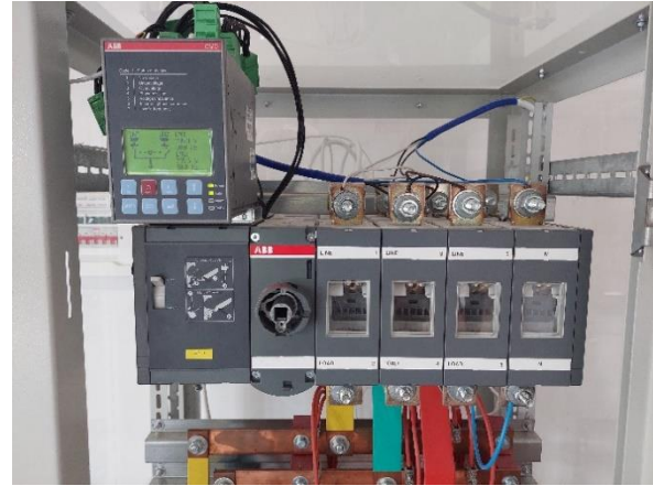
Figure 8. Reversing load switch with motor drive and automatic control unit
