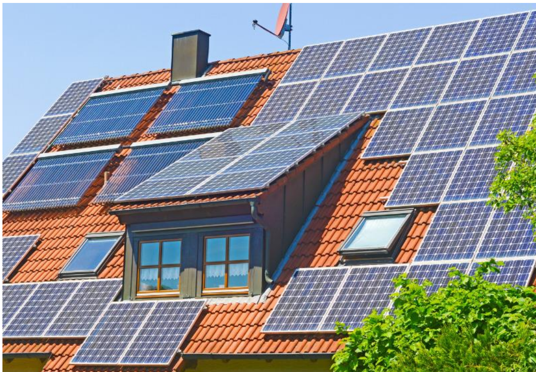
Figure 1.1 - A PV installation located on the roof of a residential building.
