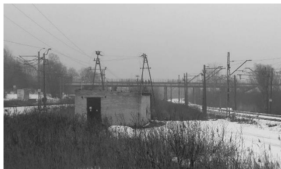
Figure 6. View of the energy installation near the railway viaduct – national road No. 15 over lines No. 353 and No. 281
