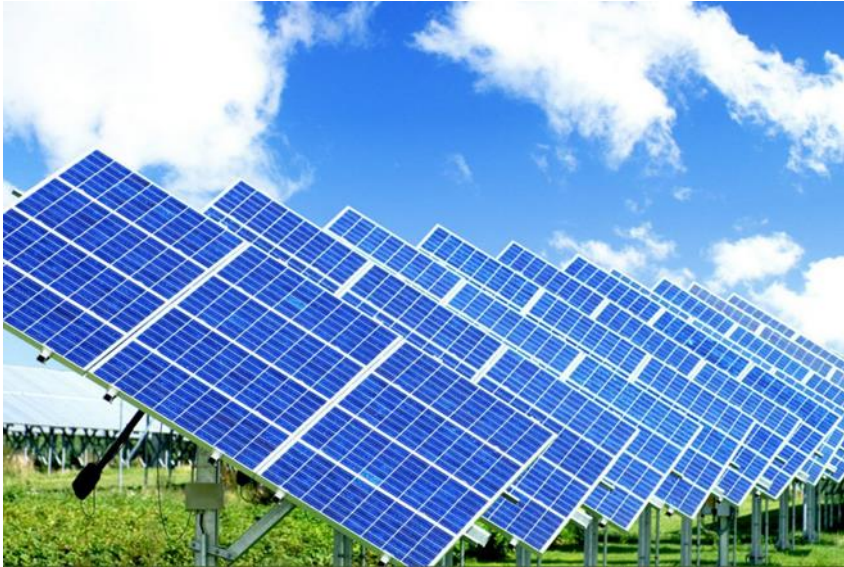
Fig. 1.3 Solar power plant
